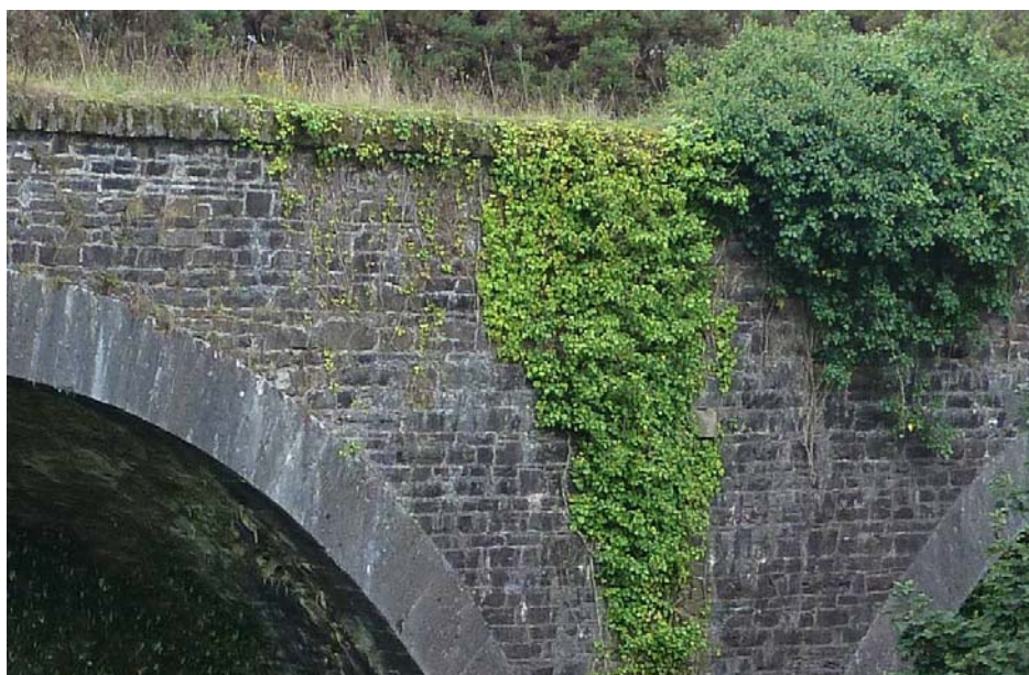
Figure 3.10: Sub surface drainage outlet in spandrel wall
