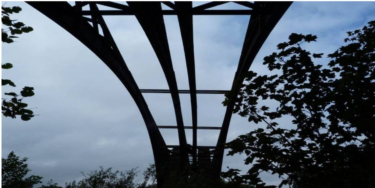
Figure 2.21: Underside of bridge deck (note absence of lateral bracing along length of arch ribs)
