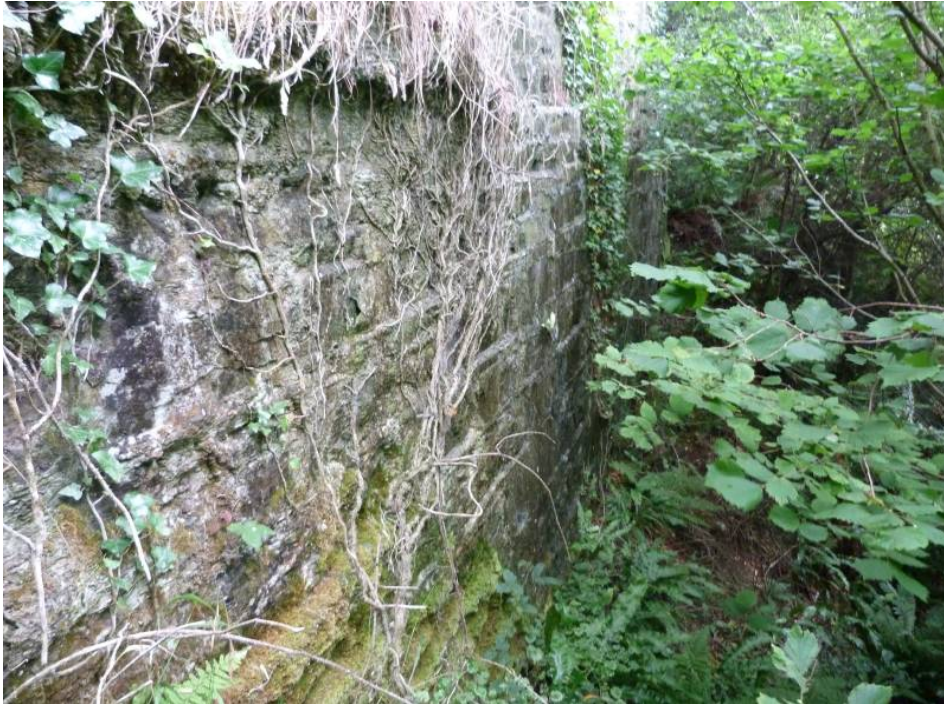
Figure 3.17: Vegetation growth on pier footing
