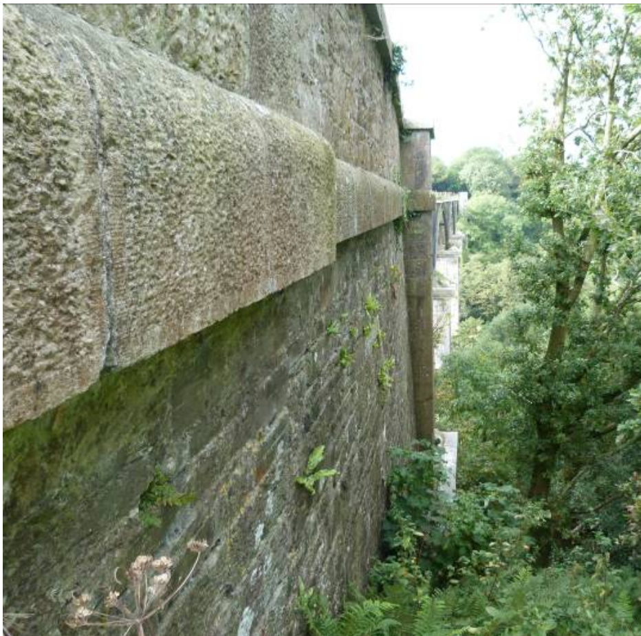
Figure 2.25: Minor vegetation growth from abutment
