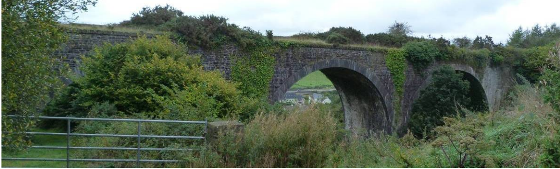
Figure 3.8: Northern elevation showing vegetation growth
