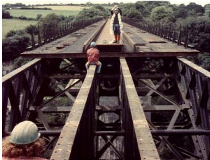
Figure 2.17: Photograph of parapet on the bridge at the time of deck removal, circa 1970
