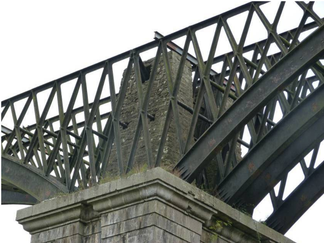
Figure 2.22: Vegetation growth on top of pier
