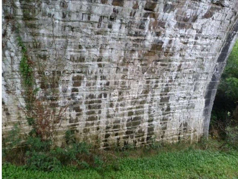
Figure 3.13: Staining to eastern abutment
