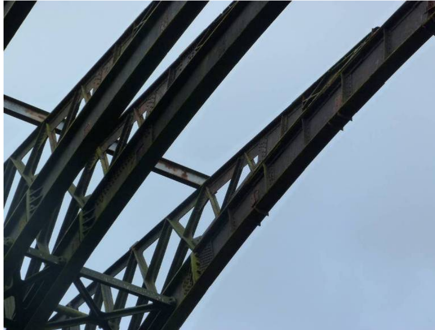
Figure 2.9: Repaired sections of arch and spandrel wall in span 3 (solid spandrel infill plates, additional stiffeners and gusset plates)
