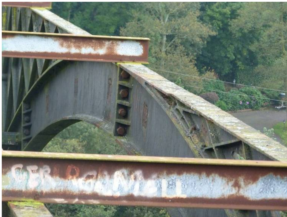
Figure 2.8: In-line bolted splice connections (note localised failure of paint system)
