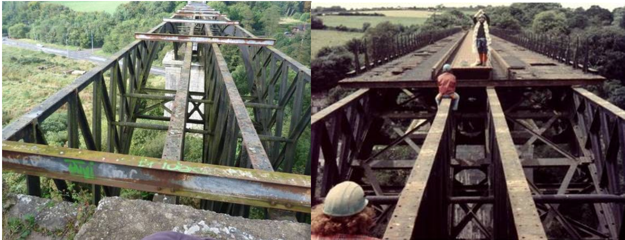
Figure 2.18: Existing condition of bracing members (left) and previous bracing members (right) during deck removal (circa 1970), note a large proportion of lateral X-shaped cast iron bracing has been removed
