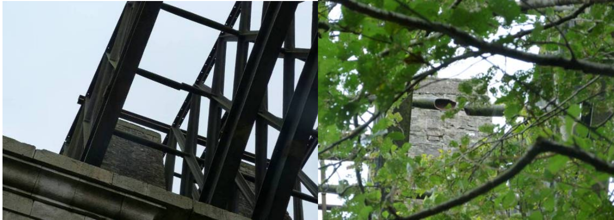
Figure 2.20: Failed wrought iron tie rods
