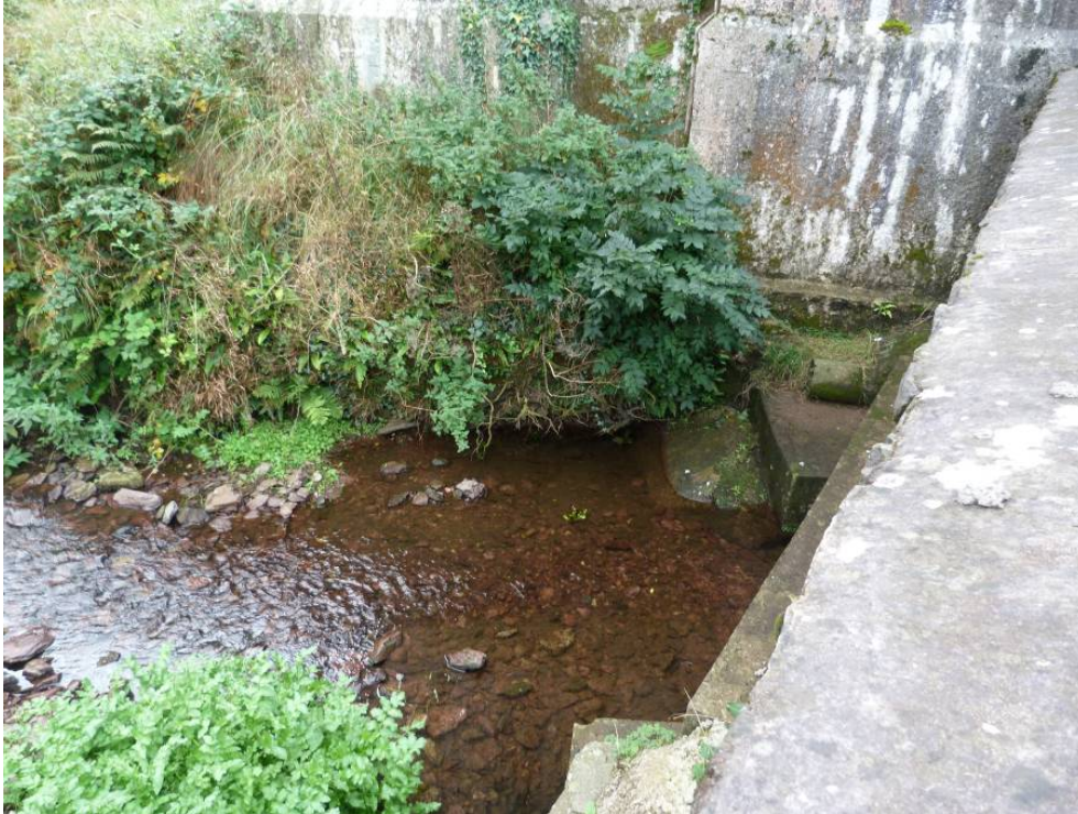
Figure 2.28: Localised erosion to the banks of the watercourse at the pier base
