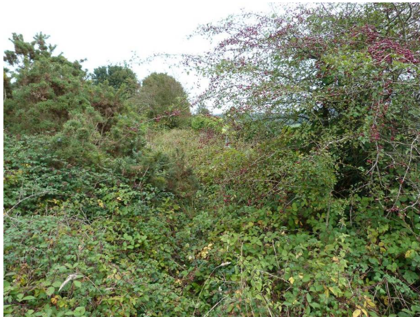
Figure 3.2: Dense vegetation growth on the bridge deck
