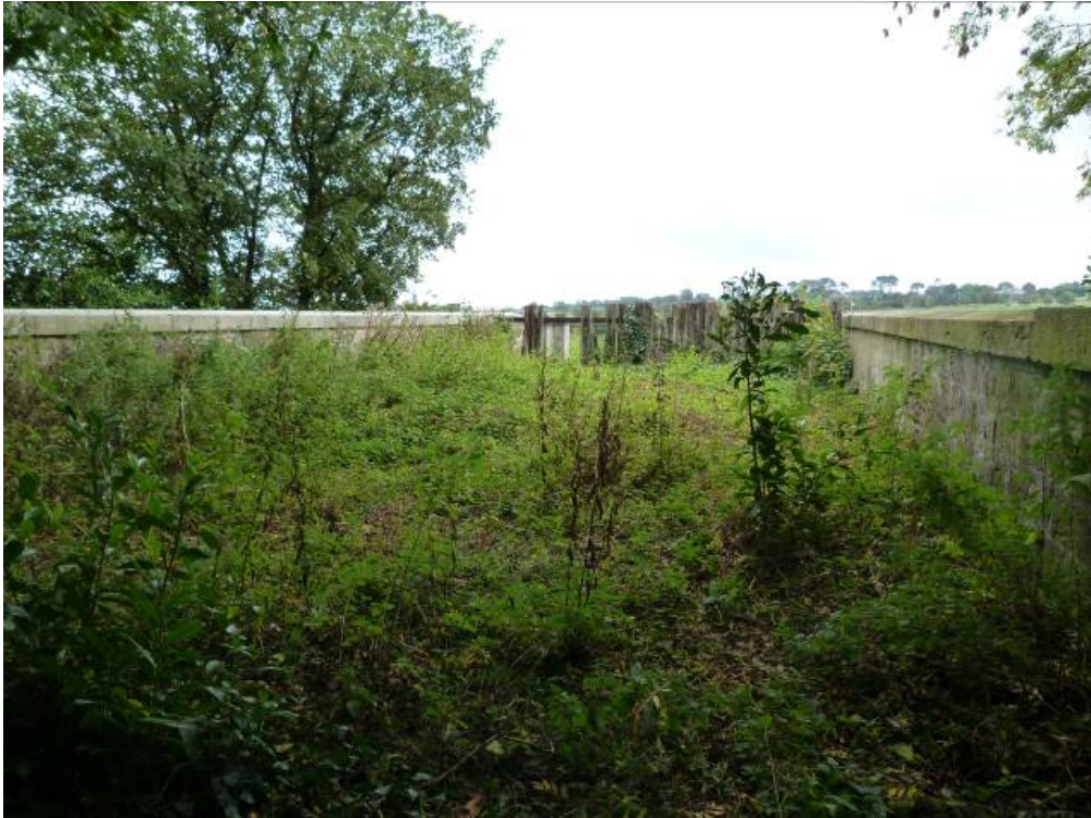
Figure 2.26: Abutment overgrown with vegetation
