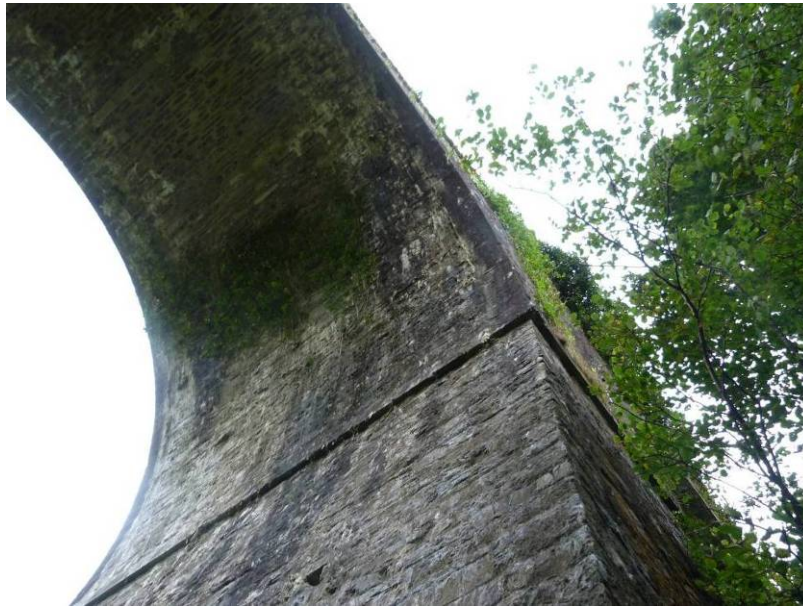
Figure 3.11: Arch barrel soffit (note water penetration)
