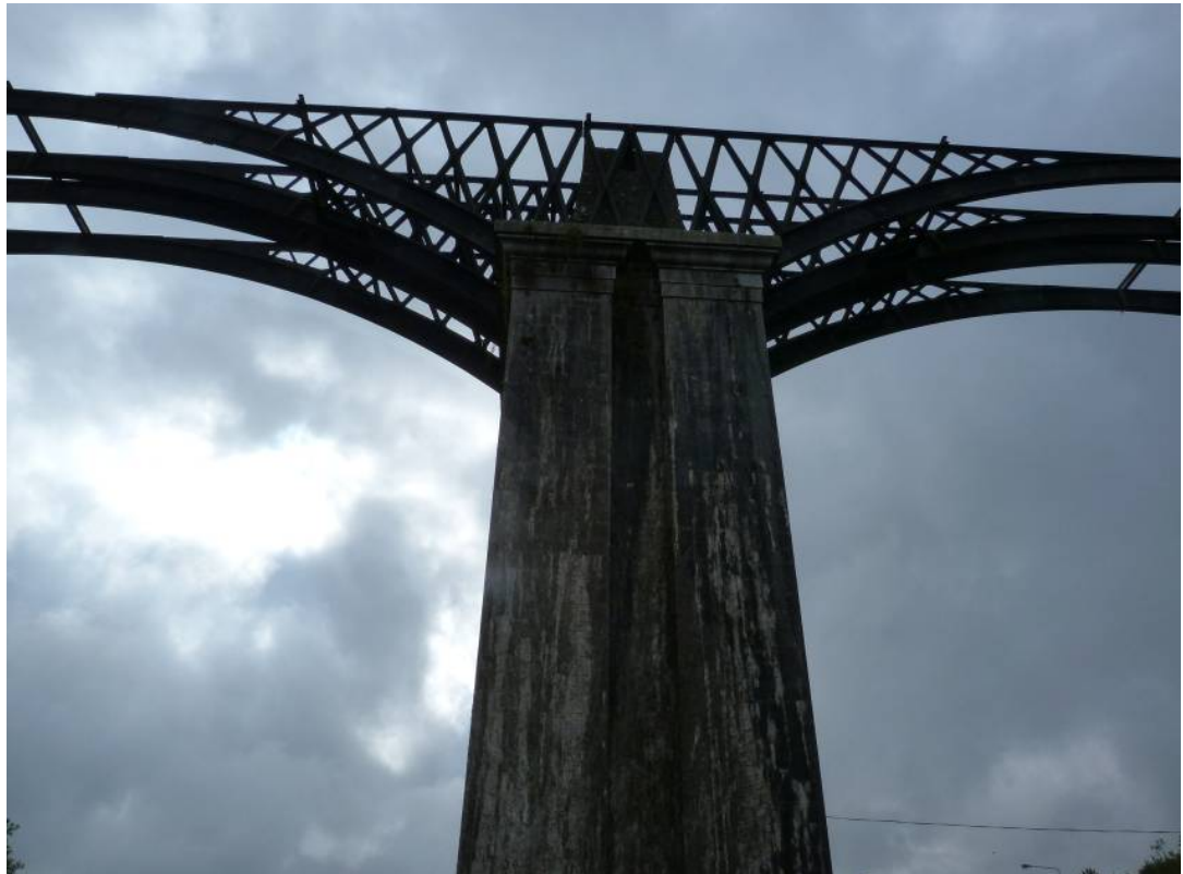
Figure 2.23: Staining on pier
