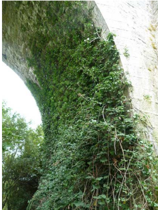
Figure 3.16: Vegetation growth on pier
